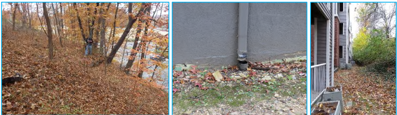
Figure 3. Evidence of enhanced downslope creep is visible throughout the slopes at the site, including leaning trees with an upwards-bending growth habit (left), displaced drain connections (center), and out-of-plumb buildings and tilted infrastructure components (right). In this unstable geologic setting, cosmetic damage to buildings may presage more serious long-term structural issues that typically appear years later. The risk of slope failures is heightened by disturbances to terrain, notably the loading of the crowns of slopes with infrastructure or artificial fill and the cutting of toeslopes for building foundations and streets. All of these risk factors are already present at the site.
